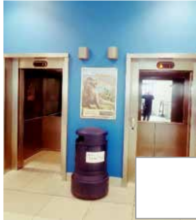
Lifts and escalators
